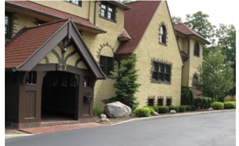
Restored entrance foyer brickwork and resealed parking lot greet the Brothers on their return.
